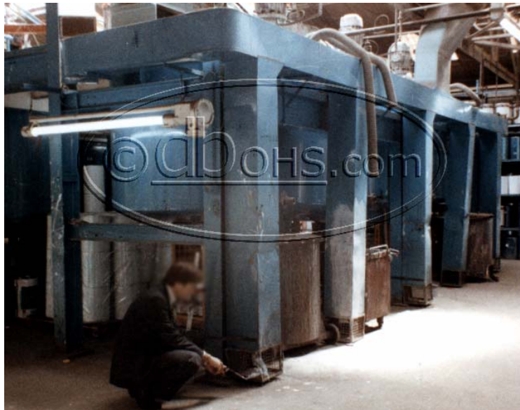
Figure 3 An expensive ventilation system at a paint factory designed to remove heavier-than-air vapours from the floor. The measured solvent concentration was uniform from the floor to at least 10 m.
